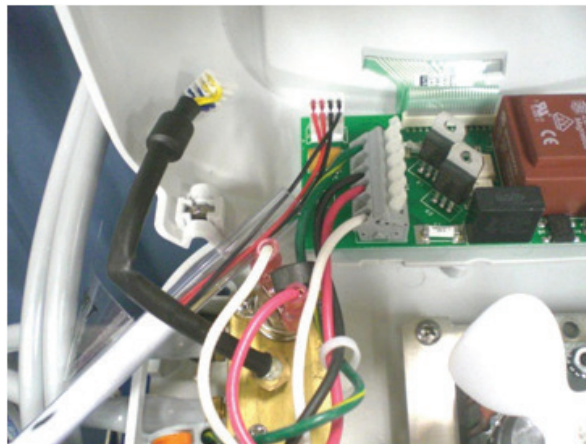
Figure 3: Connection of test temperature sensor
